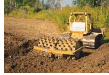
Roller Feet Embedded to Within 2 Inches of the Drum
